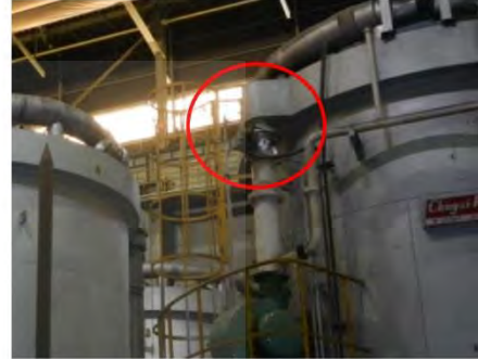
The heating cover no.24 feedback of BACV position do not stable. It effect to pressure of burner was swing.
