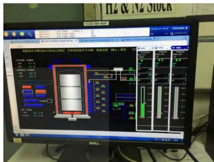
Start the heating cycle from DCS. "Code 00"
