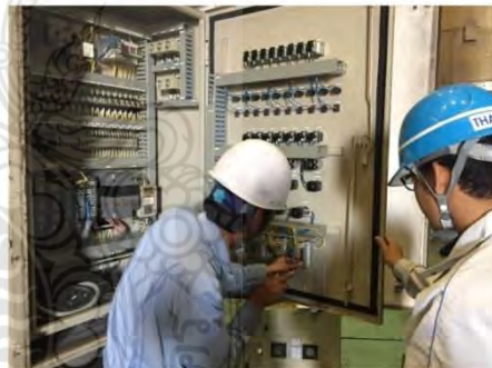
Disconnect wiring of SDC35 (BGCV).
