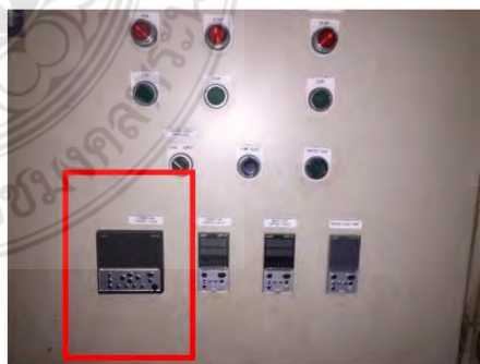
New BGCV controller after replacement.
