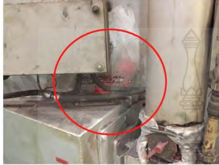
Surface was over heat of burner no. 7 at heating cover no. 4.
