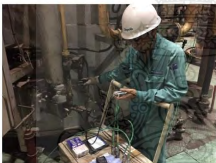
Recording data at MV value 100%, 75%, 50%, 45% and 23.1%. (Before BGCV controller replacement)
