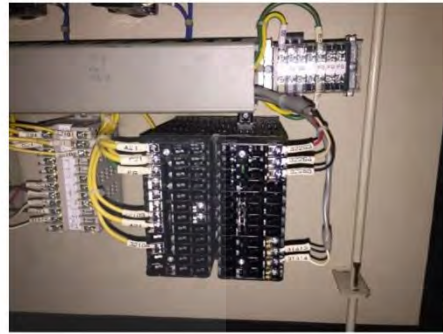
New BGCV controller wiring after replacement.
