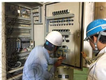
BGCV controller replacement.
