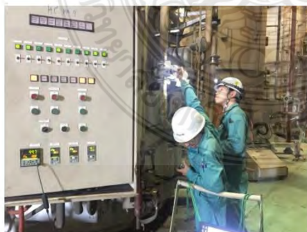
Pressure balance check and adjust combustion for each burner.
