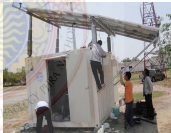
Figure.8: Construction of the designed Mobile Hybrid System
